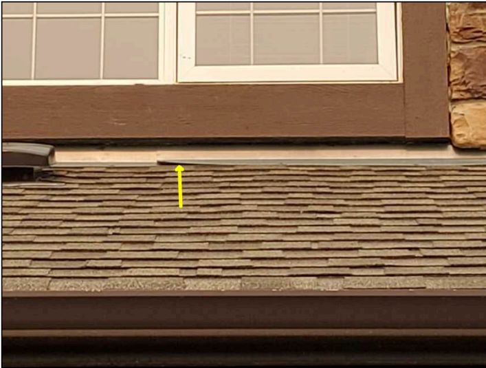
Recommend re sealing all flashing to prevent possible moisture penetration.
