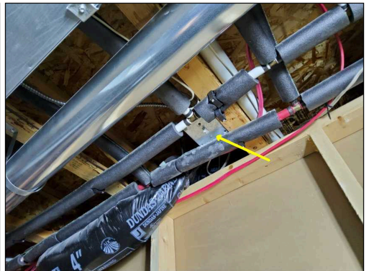
Kill switch shown to furnace - recommend relocating for easier access.
