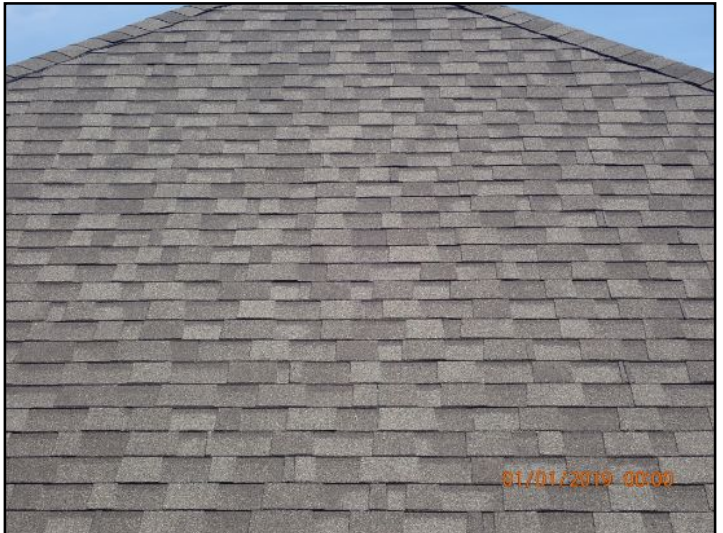
Roof appeared in serviceable condition at the time of the inspection. No prediction of future performance or warranties can be offered.
