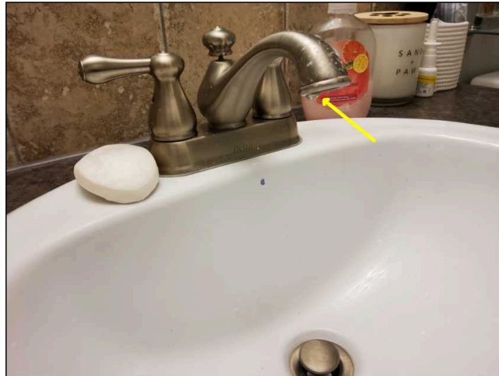
Main Bathroom - Sink Faucet drips. Repair recommended by a qualified plumber.
