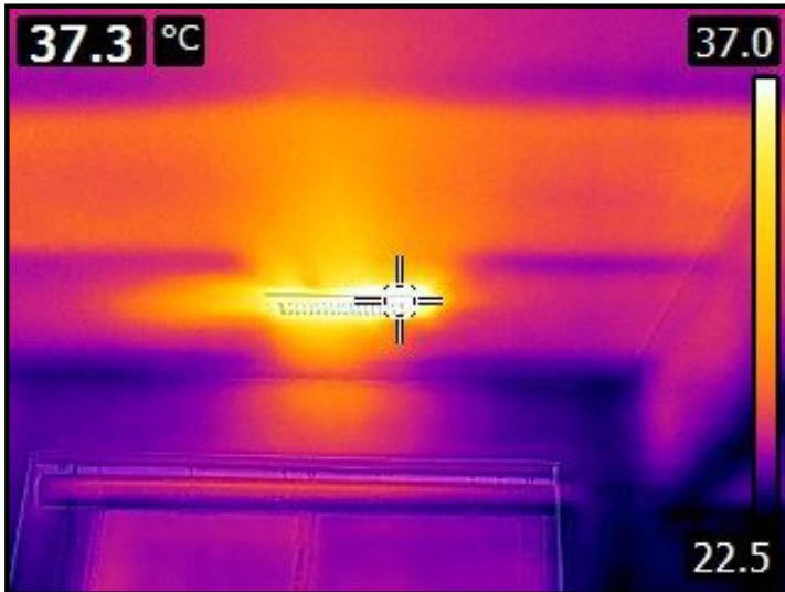
Basement bedroom heating register, responding to test
