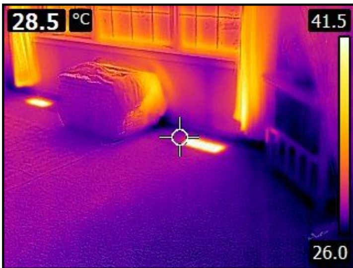
Upper level heating register, responding to test
