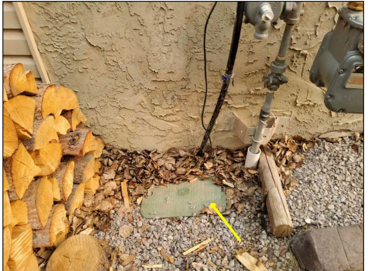
An automatic sprinkler/irrigation system was observed but not inspected or tested. This system is beyond the scope of this inspection. We recommend further review by a qualified professional, if desired.
