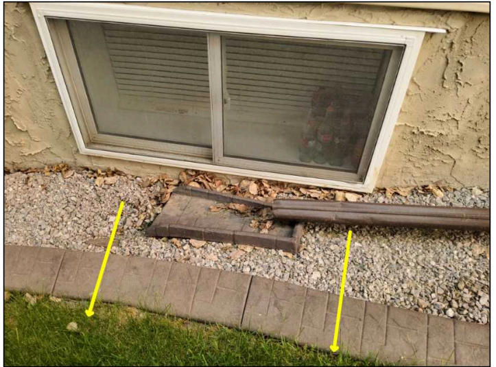
Window is at/or below grade level - recommend grading away from window or adding a window well to reduce the risk of potential water entry.
