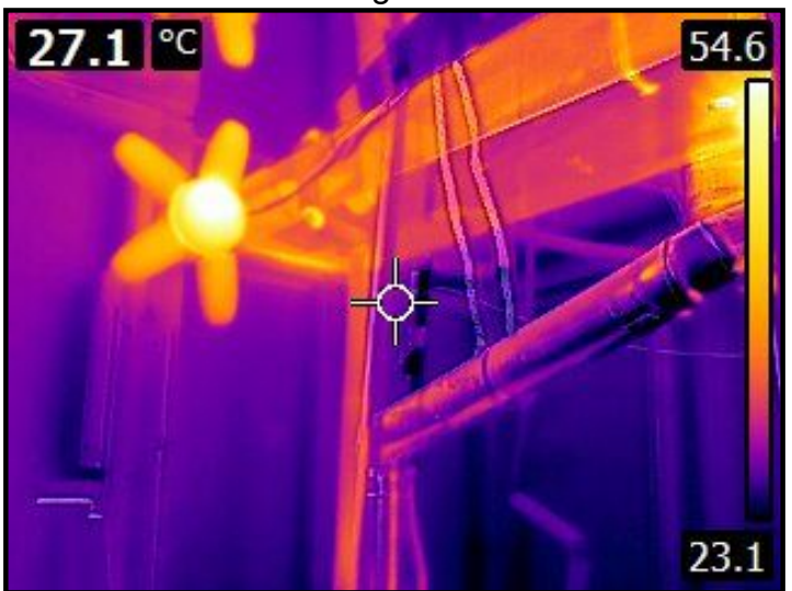
Mechanical room thermal image
