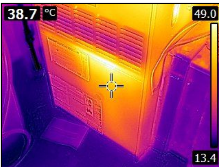
Mechanical room thermal image
