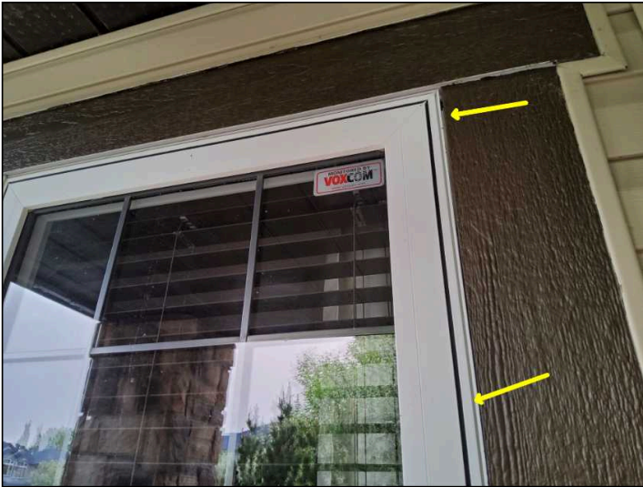
Missing and Split caulking noted maintain a good seal around all windows and doors to prevent water damage
