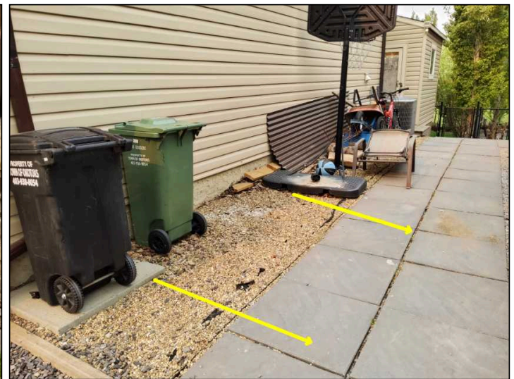
For correct drainage around the home all sides would slope away from the home, this assists in preventing water from sitting at the foundation wall.
