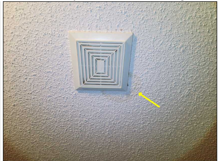
Main Bathroom - Minor staining noted around the vent fan - Water stains on the ceiling around your bath fan may indicate a leak coming from the vent cap on your roof, but condensation is the more likely culprit. If bath fan ducting is not properly insulated or there is not a loop in the line, the moist air from your house will condense inside the duct, and may run back onto the ceiling.
