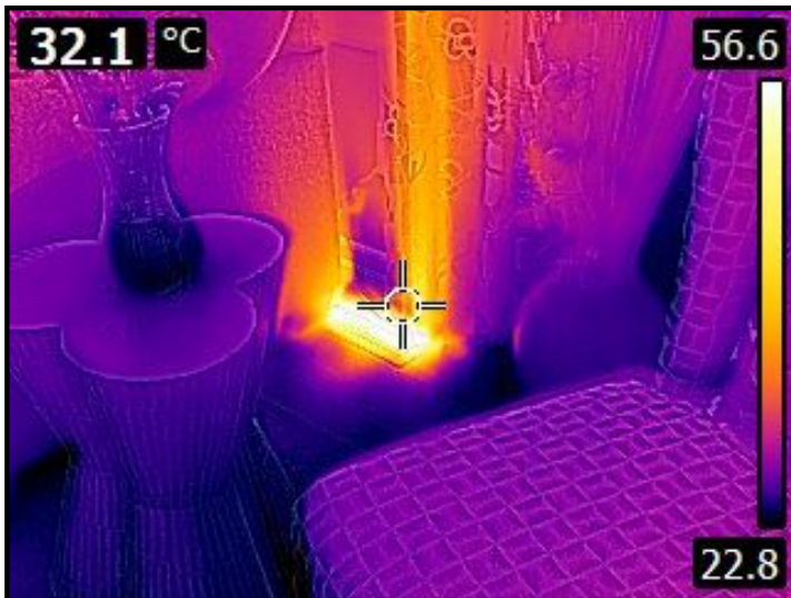
Living room heating register, responding to test
