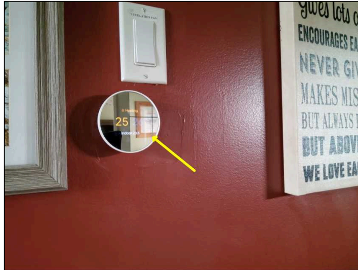
Thermostat functional on day of inspection
