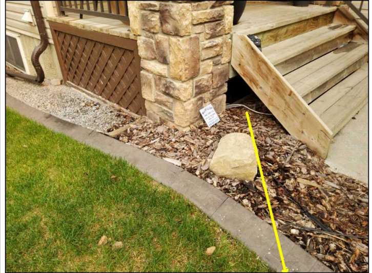
Recommend sealing gap at porch base to prevent any possible moisture intrusion and pest entry and grading away from structure.
