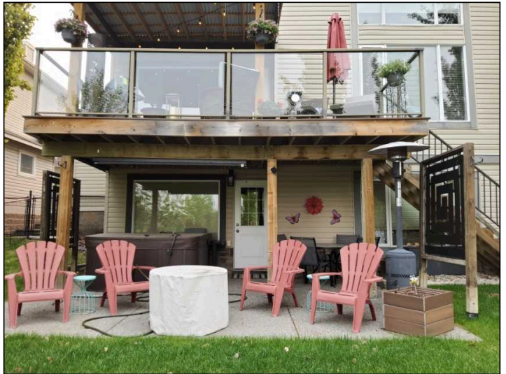
All external wood requires regular maintenance
