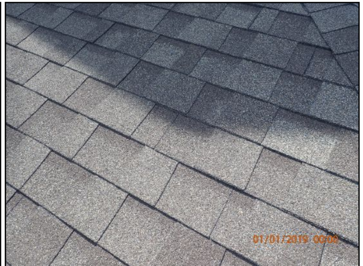
Roof appeared in serviceable condition at the time of the inspection. No prediction of future performance or warranties can be offered.
