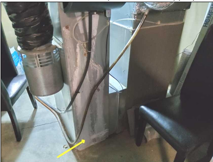
Rust and corrosion noted to the housing of this unit. Recommend inspection by a qualified HVAC contractor.
