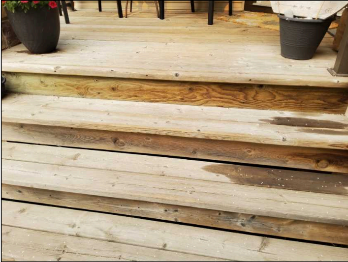
Porch is weathered, suggest cleaning, as necessary, and treating with an oil based, water-repellent preservative to protect and extend the life of the wood.
