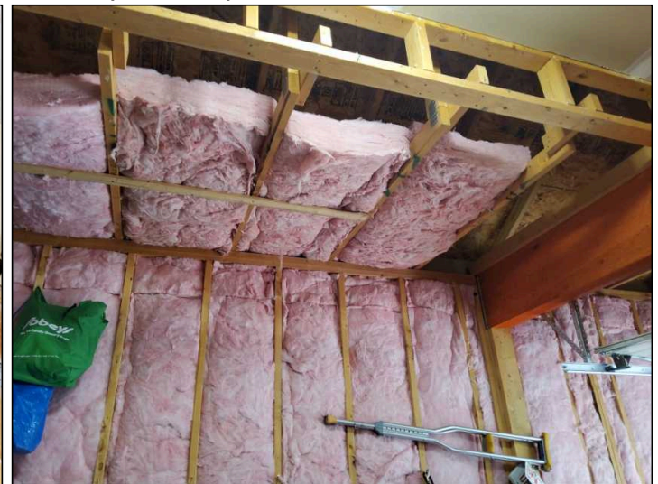
Garage partially insulated, loose insulation noted, Missing vapour barrier observed, recommend review for repair or replacement
