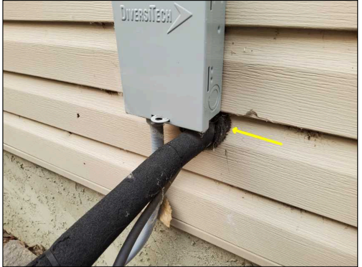
Suggest sealing/caulking as part of routine maintenance.
