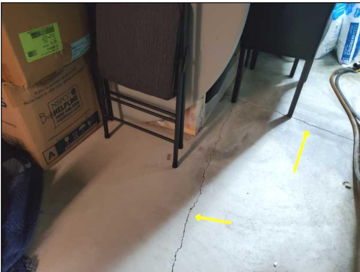
Settlement cracking noted at slab. Recommend consultation with qualified contractor should condition worsen or water intrusion occur. Recommend monitoring.
