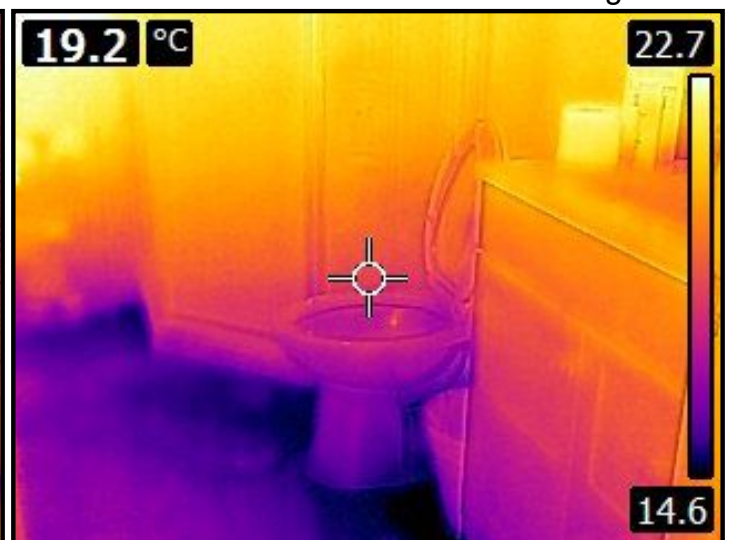
Basement Bathroom - Thermal Image
