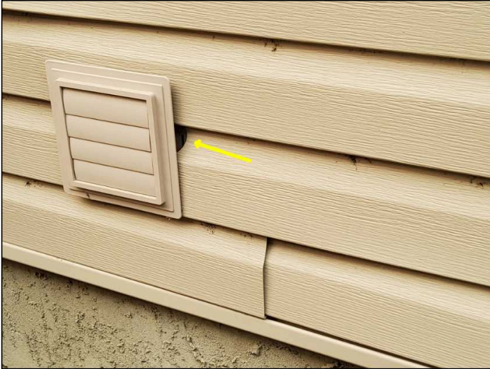
Suggest sealing/caulking as part of routine maintenance.
