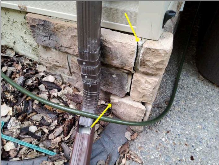
Damaged loose stone cladding observed, recommend review for repair or replacement
