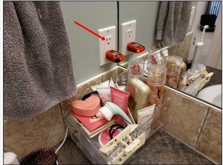
Main bathroom receptacle did not trip en suite GFCI, recommend review by a certified electrician
