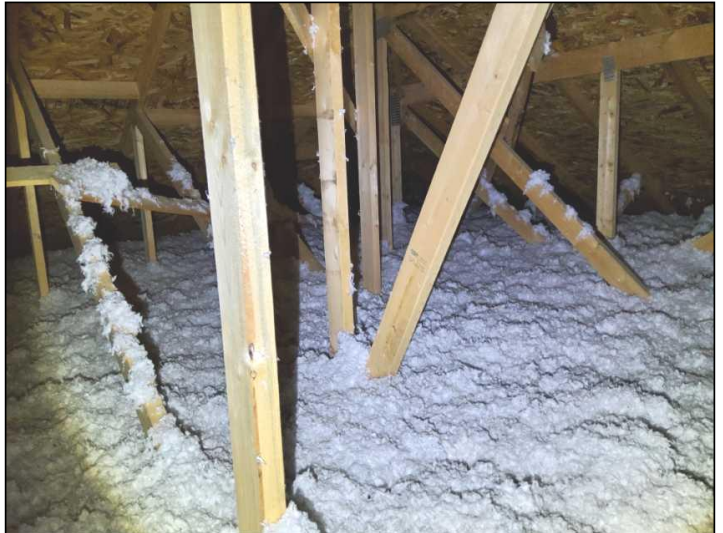
Unable to determine condition in some areas due to framing and insulation cover.
