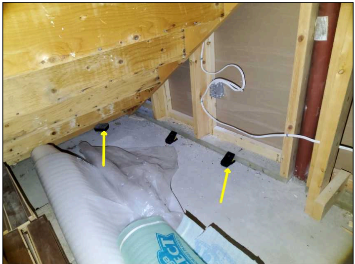
Indication of possible pest activity observed, recommend further review by a certified pest control if concerned
