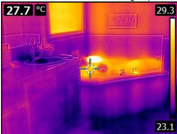
En Suite to Primary Bedroom - Thermal Image
