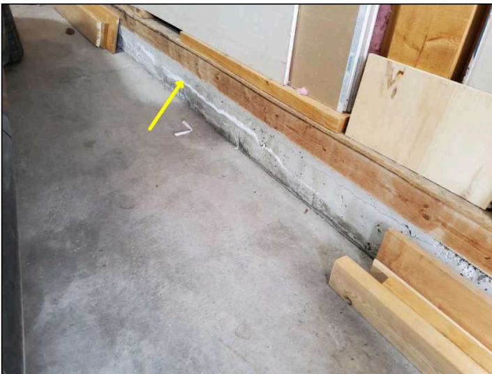
Efflorescence observed; this is a mineral deposit left behind from exterior water infiltration and vehicle snow melt off.
