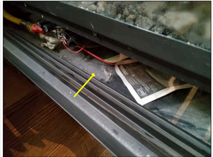
Recommend servicing and cleaning by a contractor.
