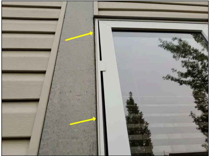
Missing and Split caulking noted maintain a good seal around all windows and doors to prevent water damage
