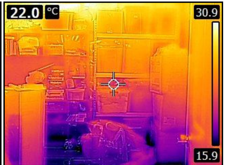
Limited thermal scan due to storage of personal property. Recommend further review prior to close or final walk through.
