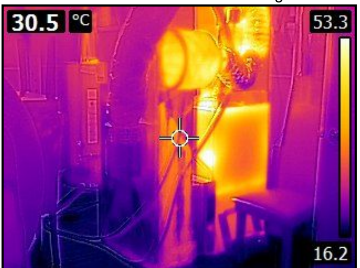
Mechanical room thermal image
