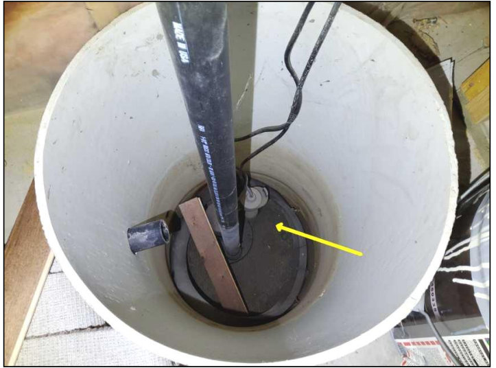
Unable to test due to a dried pit with no external switch. Recommend client confirm proper operation prior to close.
