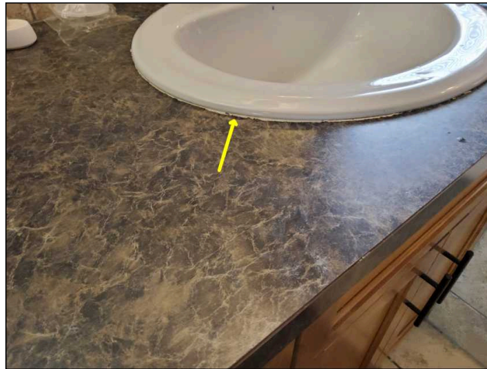
- Recommend caulking as necessary.
