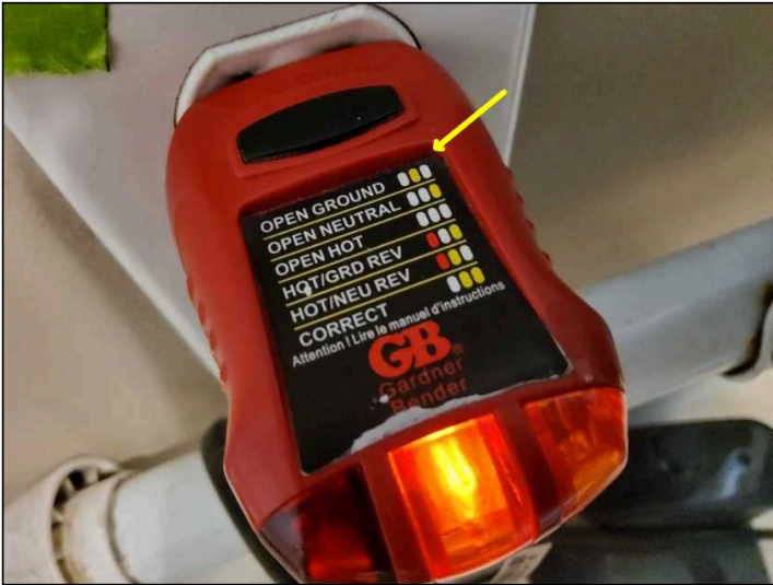
Multiple open grounded receptacles observed. Recommend further assessment by a certified electrician.
