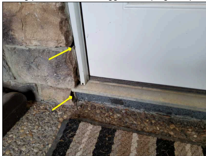
Missing and split caulking observed, recommend resealing as part of the ongoing maintenance
