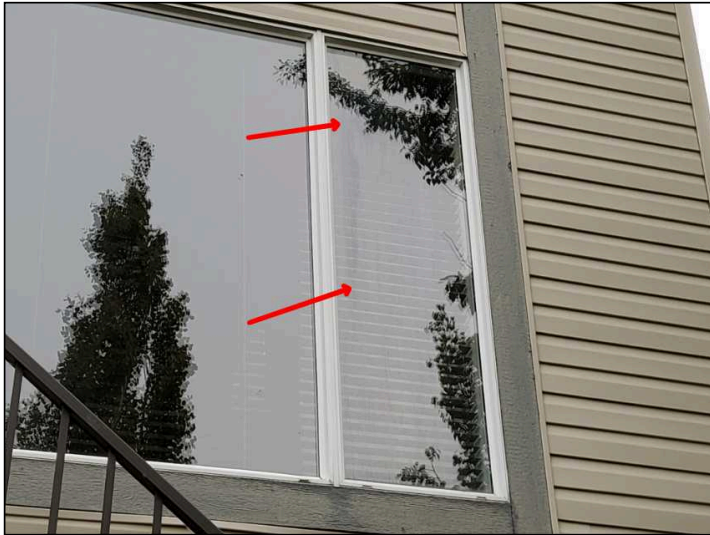
Fog/condensation observed in thermopane windows. This is an indication of a failed seal. Recommend review for repair or replacement as necessary.
