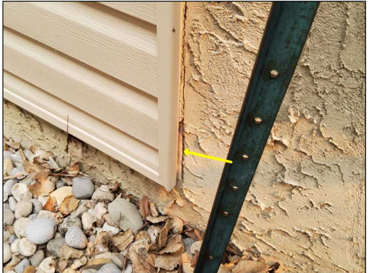
Suggest sealing/caulking as part of routine maintenance.
