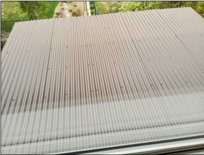
Metal Roof appeared in serviceable condition at the time of the inspection. No prediction of future performance or warranties can be offered.
