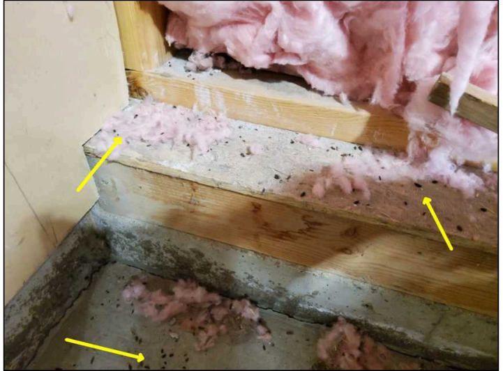
Indication of possible pest activity observed, recommend further review by a certified pest control if concerned
