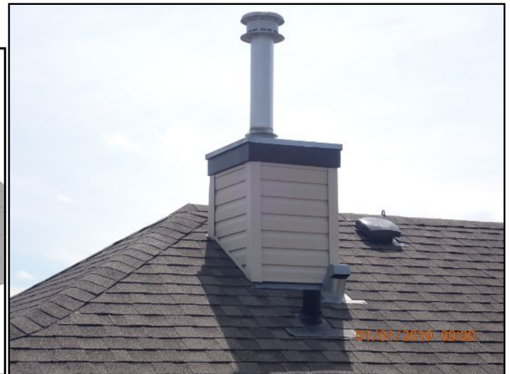
Chimney is in serviceable condition where visible - Ongoing monitoring and maintenance required.
