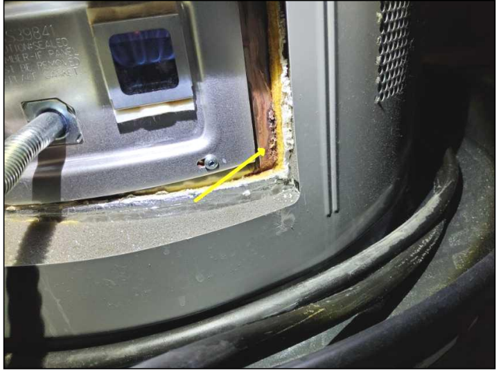
Rust and scale noted to combustion chamber
