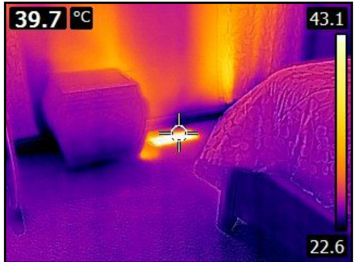
Bedroom heating register, responding to test.
