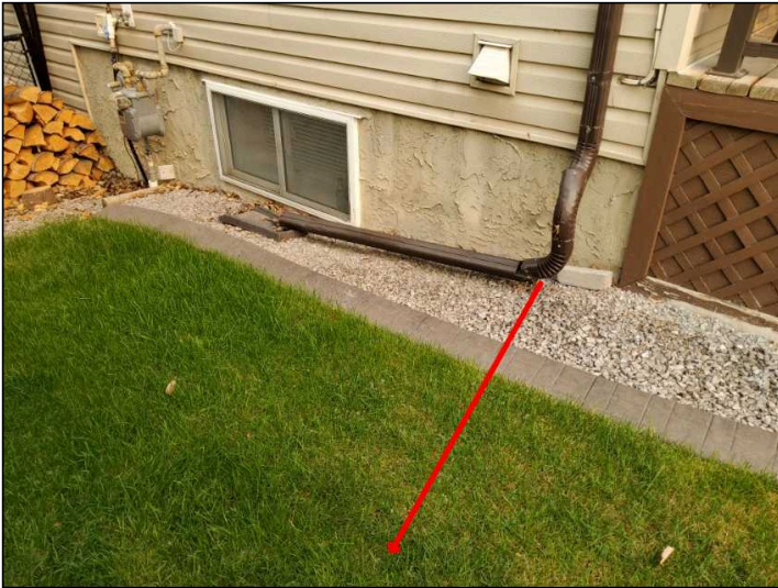
Extend downspouts 5-6 feet from the foundation of the home for effective water flow.
