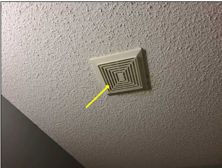
Fans are dirty and requires cleaning
