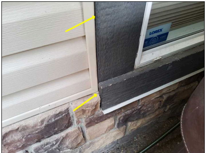
Suggest sealing/caulking as part of routine maintenance to prevent deterioration.
