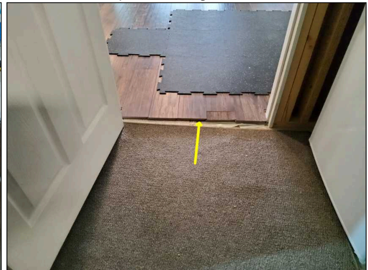
A sub floor has been added. Unable to inspect the original slab.
